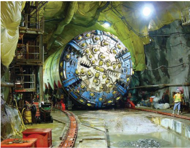
Las Vegas built its own intake tunnel to draw water from the lowest depths of Lake Mead even during drought. Brierley Associates used a custom-built drilling machine to dig out the tunnel. Photo credit: Brierley Associates
