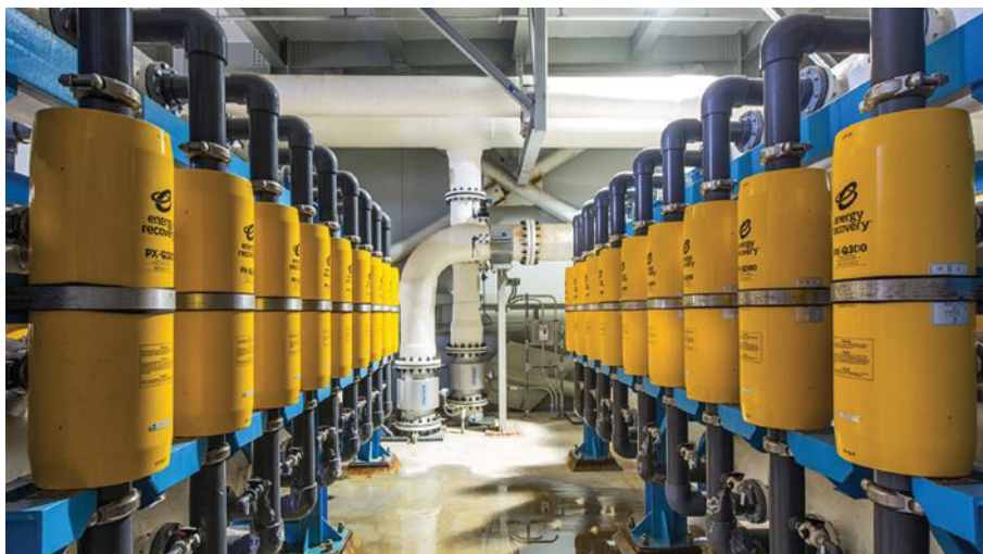
Pressure recovery modules at Poseidon Water’s Carlsbad desalination plant in San Diego County. Photo credit: Poseidon Water
