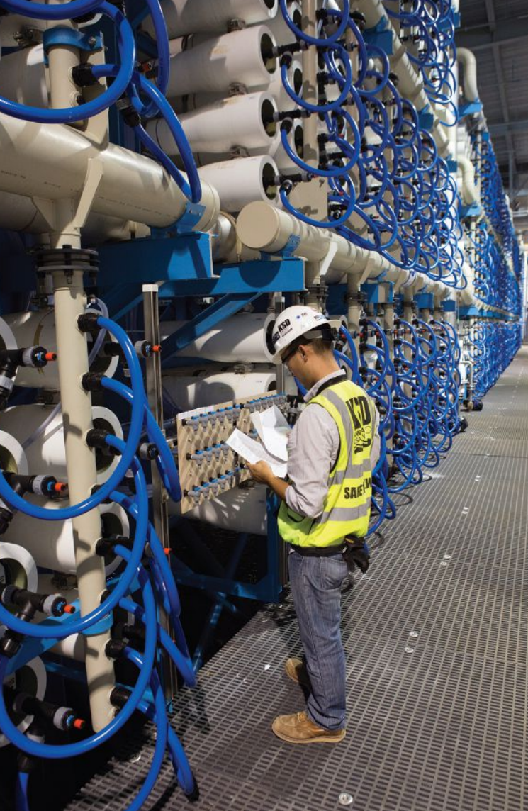
Pressure vessels containing reverse osmosis membranes are the heart of the Carlsbad Desalination Plant, to start supplying 8 percent of San Diego County with desalinated ocean water by mid-2016. Photo: Poseidon Water
