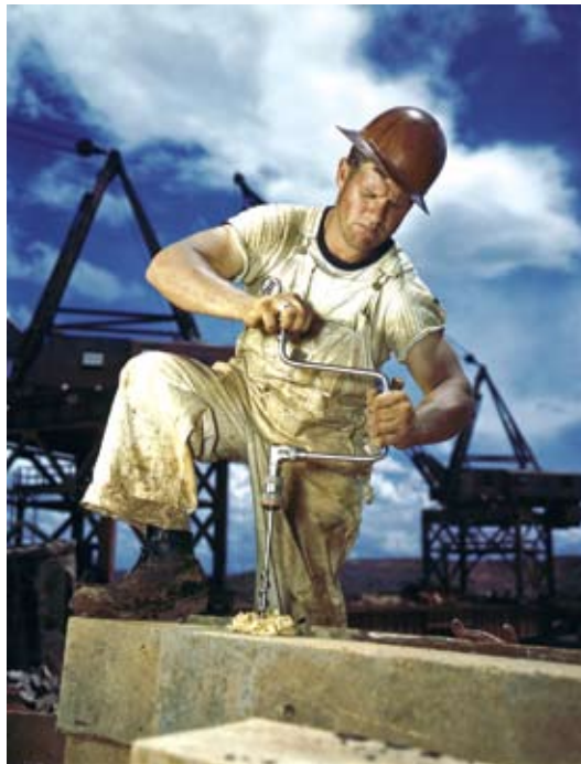
A construction site carpenter at work in 1942 on the TVA’s Douglas Dam in Tennessee.
