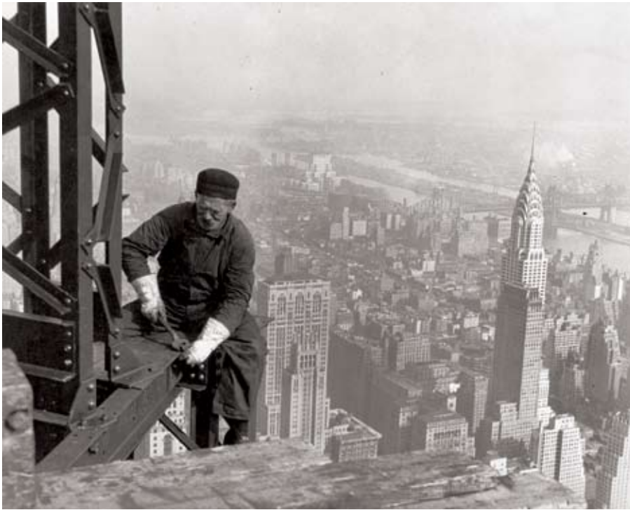
A construction worker installs girder bolts on New York City’s Empire State Building in 1931, with the Chrysler Building shown behind.
