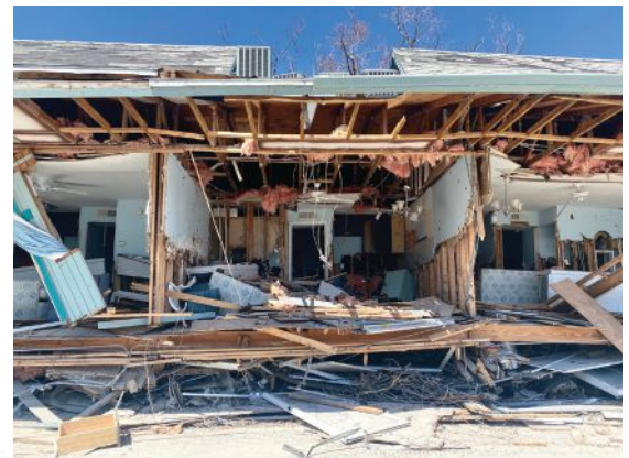
Hurricane Andrew's 157 mph winds ripped apart this home when it drove through Florida and Louisiana.
