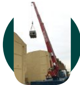
Michael Payne postponed installing his new HVAC system to support WV Beta students. Image of the delayed installation above.
