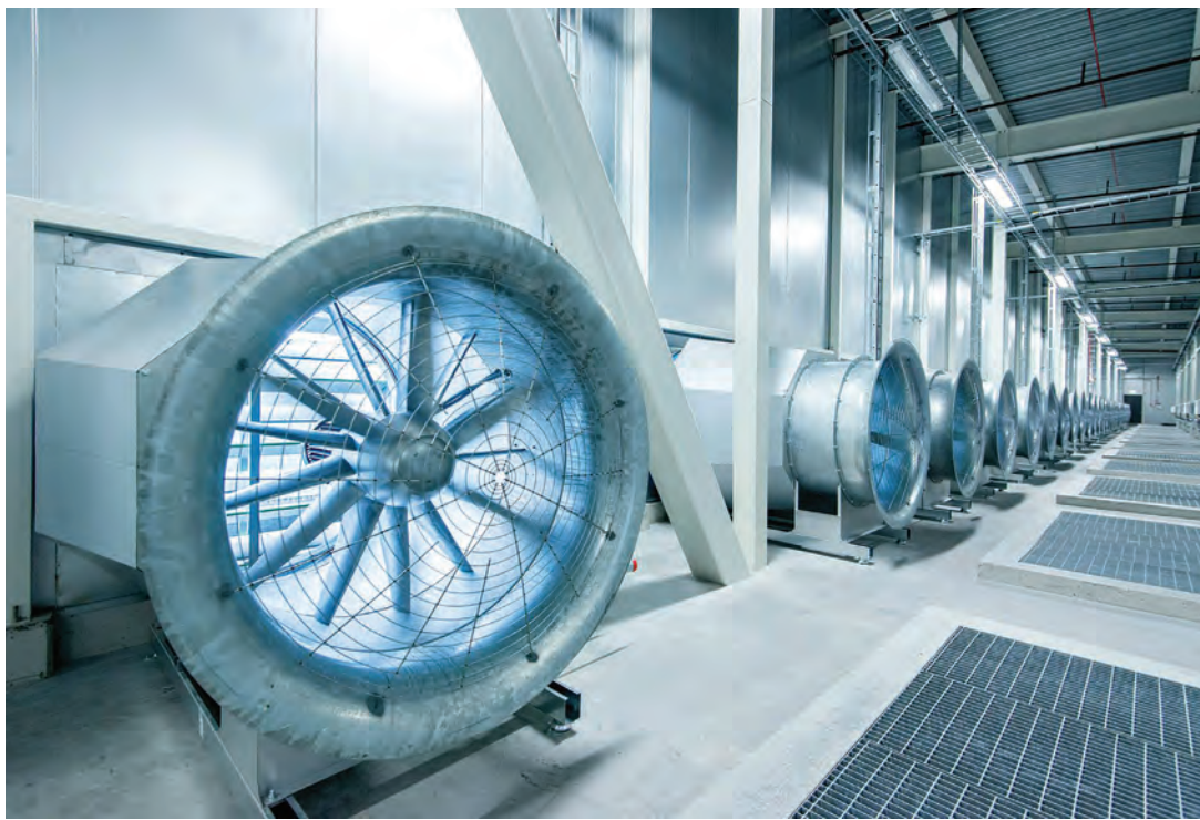
Cooling fans at the Facebook data center at Lulea in northern Sweden. Photo: Facebook
