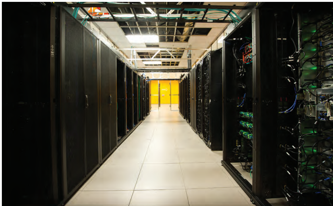
Inside the hot aisle containment racks in the high performance computing data center at NREL's Energy Systems Integration Facility. Photo: Dennis Schroeder/NREL
