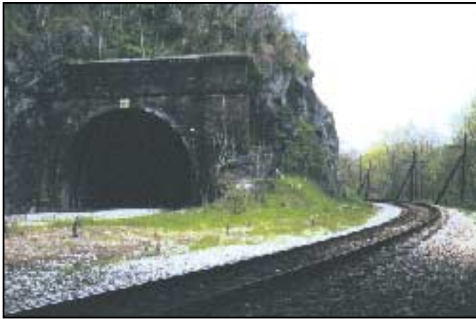
The final insult. When the new longer and taller railway cars wouldn't fit through the old double-track tunnel at Point of Rocks, one track was moved to the center of the tunnel and the now-defunct canal filled in for the other (milepost 49).
