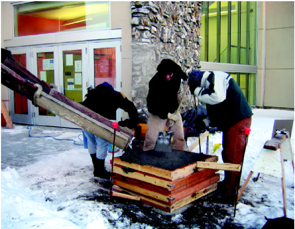
Margaret Darrow, Nathanael Vaughan, and Ben Dobrovlny (left to right) work concrete into its form in sub-zero temperatures.
