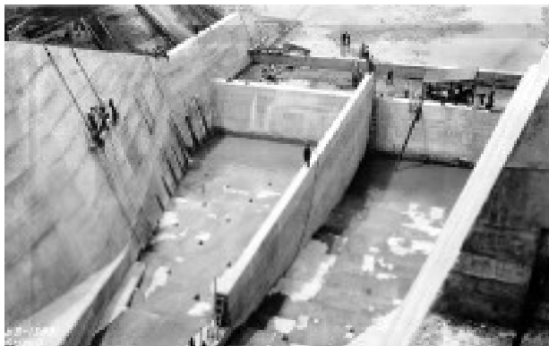
Stilling pool at the base of the spillway (left) is viewed from the top of the Lockington Dam, the northernmost dam of the Miami Conservancy District near Piqua, OH, looking downstream (water would flow toward the upper right). Stair-step structures on the spillway's floor, as well as the wall at the end, are part of the hydraulic jump used to dissipate high-velocity water's kinetic energy under flood conditions. In the photograph taken June 11, 1919, construction equipment is being
