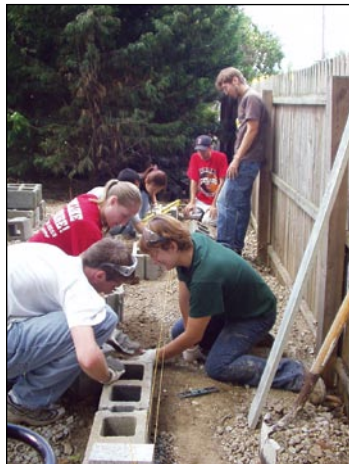
Laying the large shed's foundation gave Tau Bates an opportunity to put familiar engineering principles into practice.
